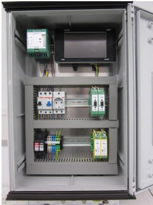
Figure 6: Example of a Standard Lufft UMB Control Cabinet
