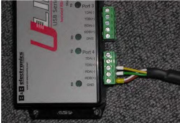
Figure 13 RS485 connection to transducer.
